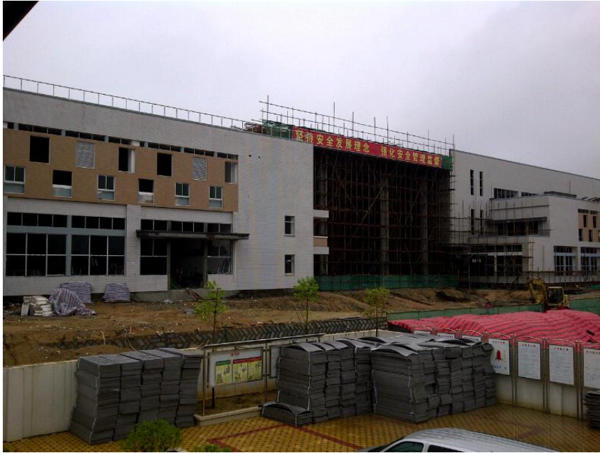
Phase 1 of production block nearing completion during Australian directors' site visit on 5 September.
